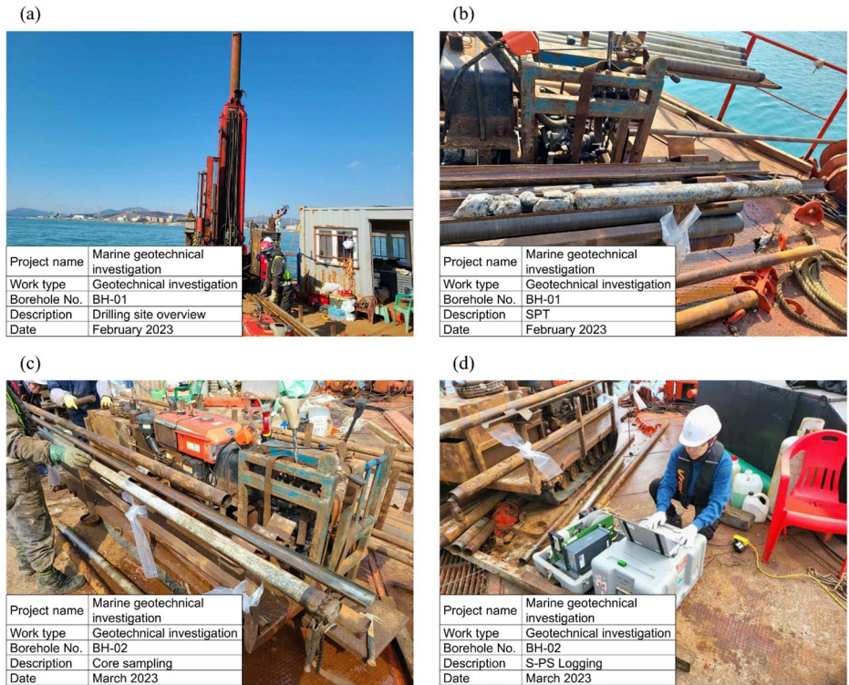
Fig. 2 Overview of borehole investigation activities: (a) general overview of drilling operation at BH-1, (b) standard penetration test (SPT) at BH-1, (c) core sampling at BH-2, and (d) S-PS logging at BH-2
