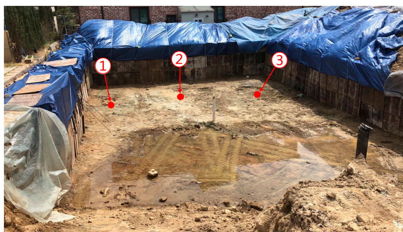
Figure 2. Measurement locations of thermal conductivity on going-to-build basement floor. The Numbers (i.e., ①, ②, and ③) mean the thermal conductivity measurement locations.
