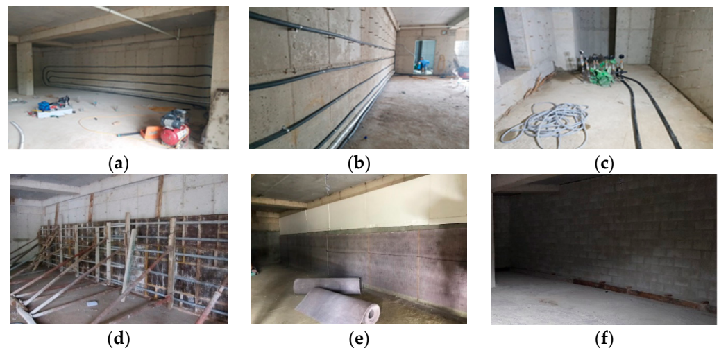
Figure 7. Construction procedure of wall-type energy slab. (a) Arrangement of heat exchange pipes. (b) Fixing heat exchange pipes. (c) Connection of supply and return pipe. (d) Placement of concrete on wall slab. (e) Installation of aerogel-type thermal insulation. (f) Placement of cement mortar and installation of bricks.
