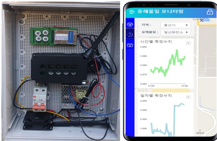
Figure 4.17 Industrial field installed IoT edge computing device and its monitoring result.
